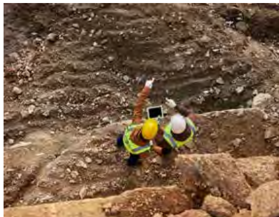
Construction workers inspecting site using digital tablet. Photo: Seventy Four © Getty images
